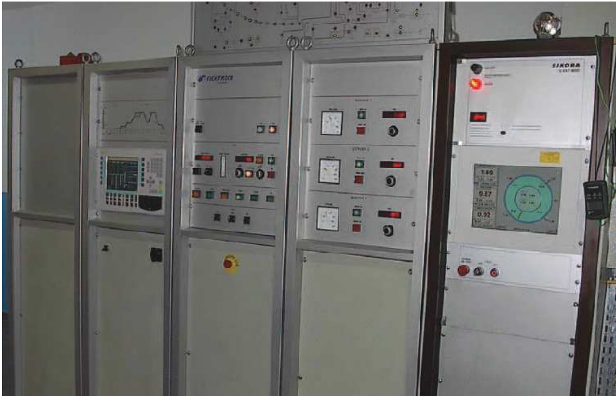
Control Panels show readouts for dimension, temperature, line speed and various other feedbacks
