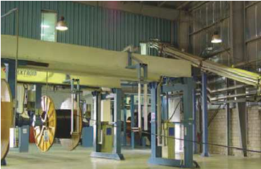
View of the CV-Lines tube that cross link the PE through dry or nitrogen curing
